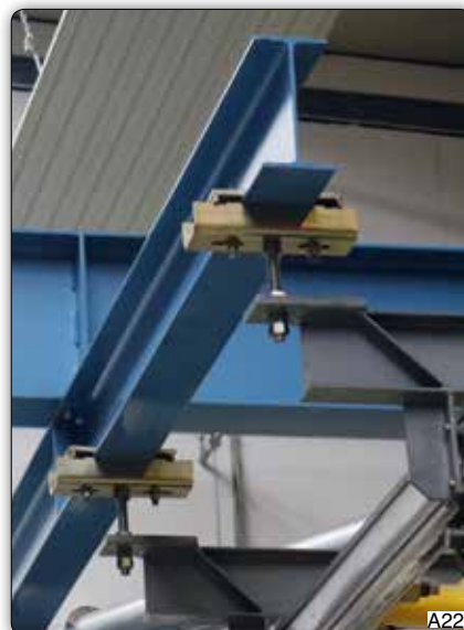
Runway suspension brackets
